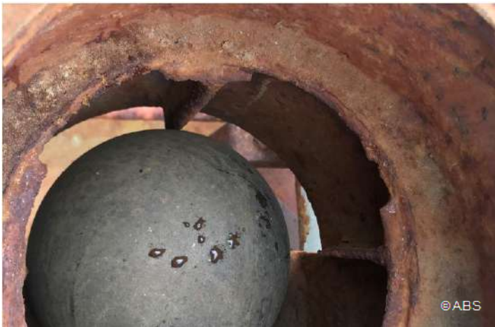
Tank vent head ball is stuck and not making positive seal, due to damaged structure
