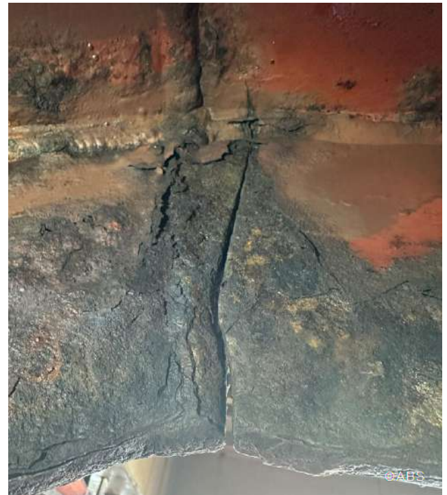
Cargo hold coaming stiffener fracture
