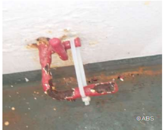
Man Overboard Buoy (MOB) unable to release due to operating mechanism stuck caused by wasted handle
