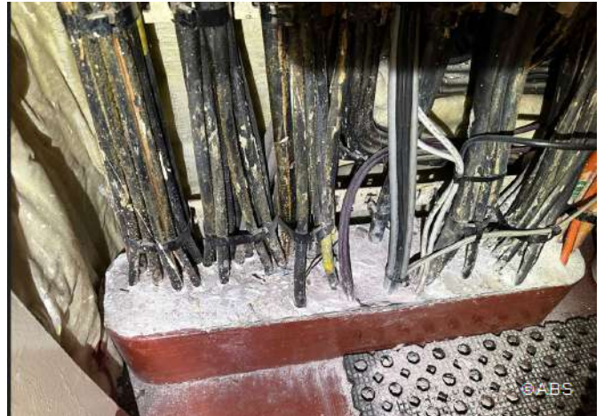
Improperly installed or modified, cable penetrations and sealing compound materials
