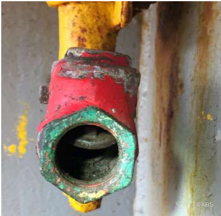
Cargo hold hatch drainage pipe valve stuck in open position
