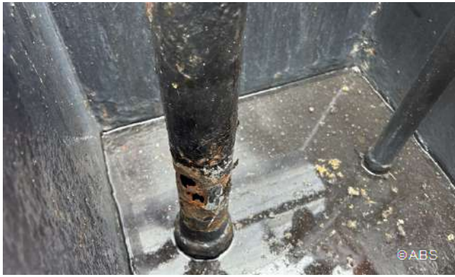
Emergency generator fuel oil tank, air vent pipe wasted with holes and covered with tape
