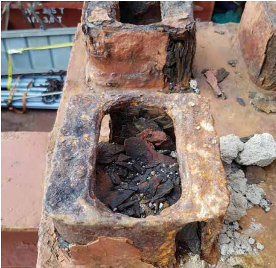
Figure 3 – IACS is developing Unified Requirement C8 to enhance the wear, tear, and corrosion of container stowage and securing systems
