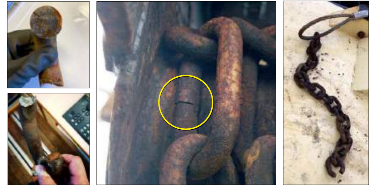
Figure 3: Identified chain defects in static pin arrangements
