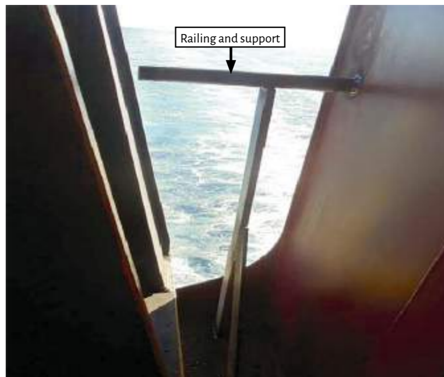
Figure 2: The guarded opening following remedial action
