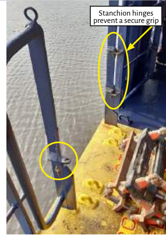
Figure 4: An access gate without suitable stanchions for the pilot to gain a secure grip
