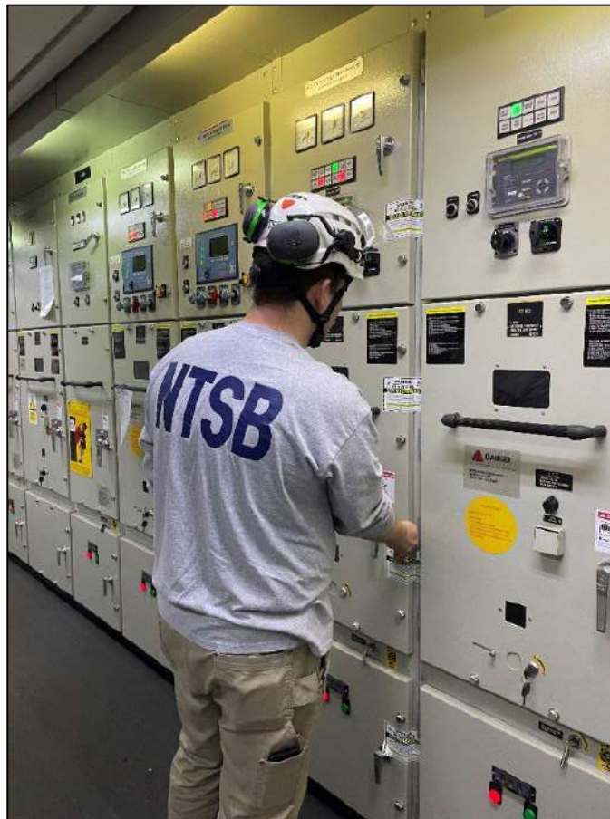
Figure 8. An NTSB investigator examining the Dali 's HV switchboard (which houses the HV bus) and applying tamper-evident preservation seals.
