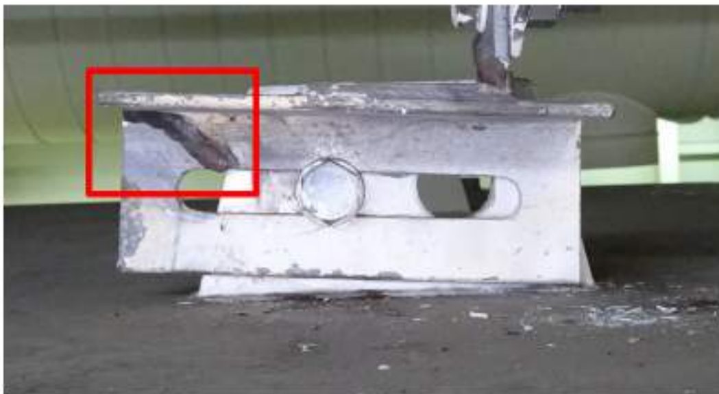
Cracked steel bracket with weld repair at the number 1 step-down transformer.
