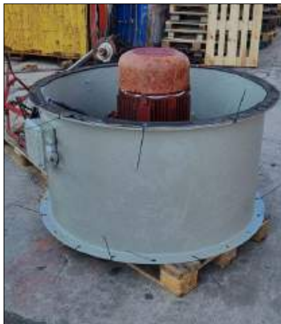
Figure 8: Starboard engine room fan unit awaiting replacement on board
