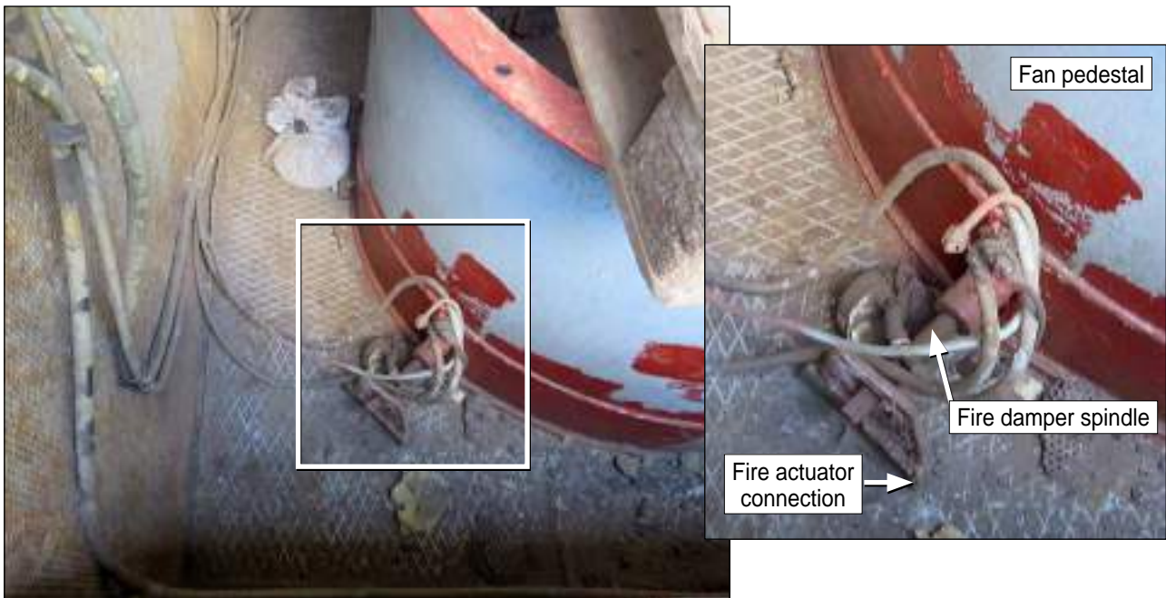
Figure 6: Disconnected fire damper actuator
