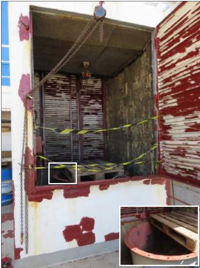
Figure 7: Painting work on the starboard fan room, showing the areas of red and pink primer paint applied by the deck crew
