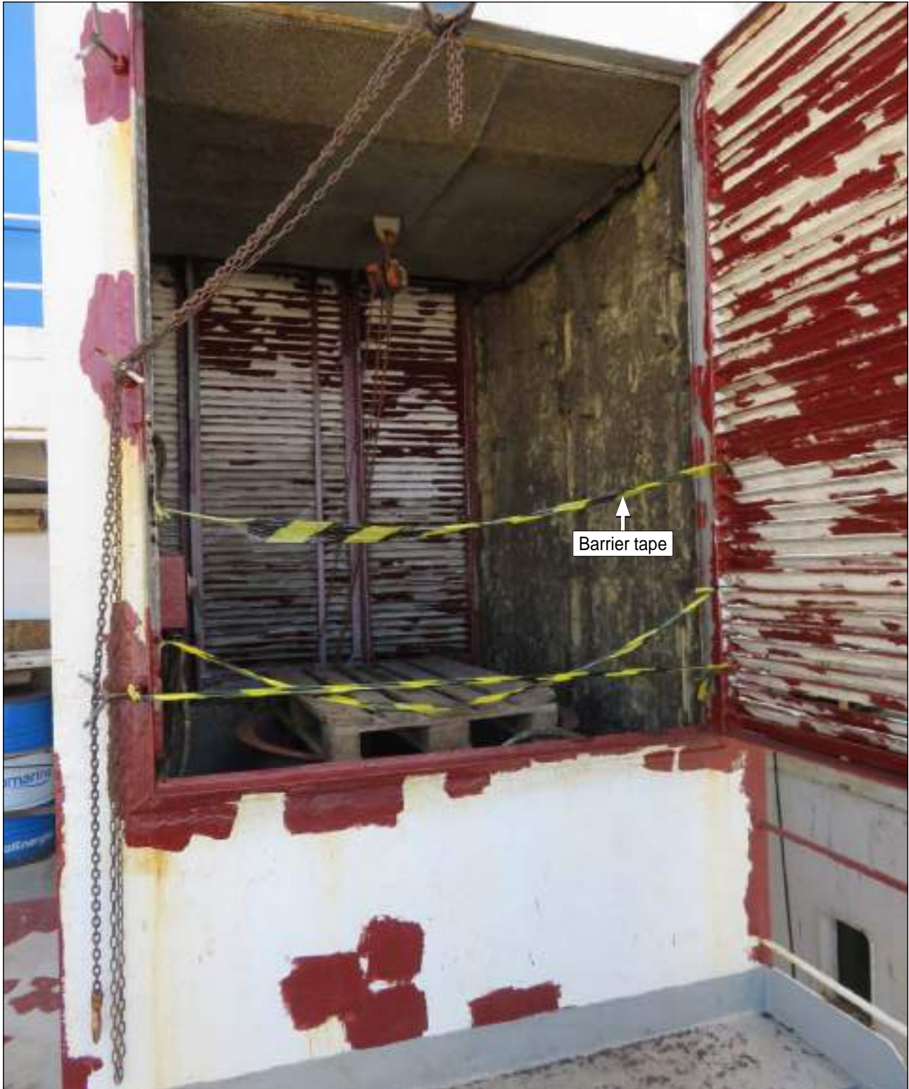
Figure 9: Barrier tape across the fan room access
