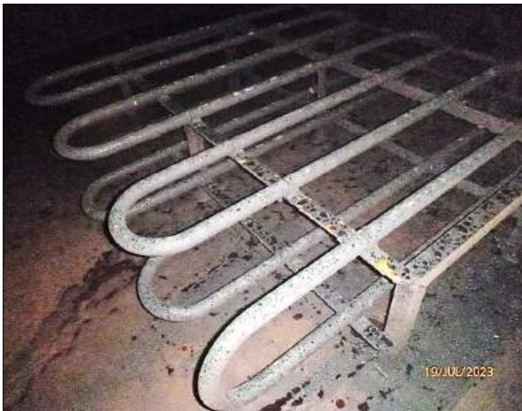
Figure 5: Photograph of the clean and dry slop tank
