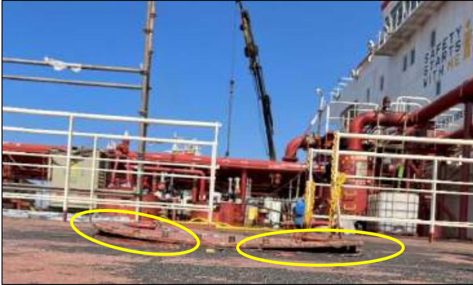
Figure 10: Buckling of the port side slop tank's manhole cover
