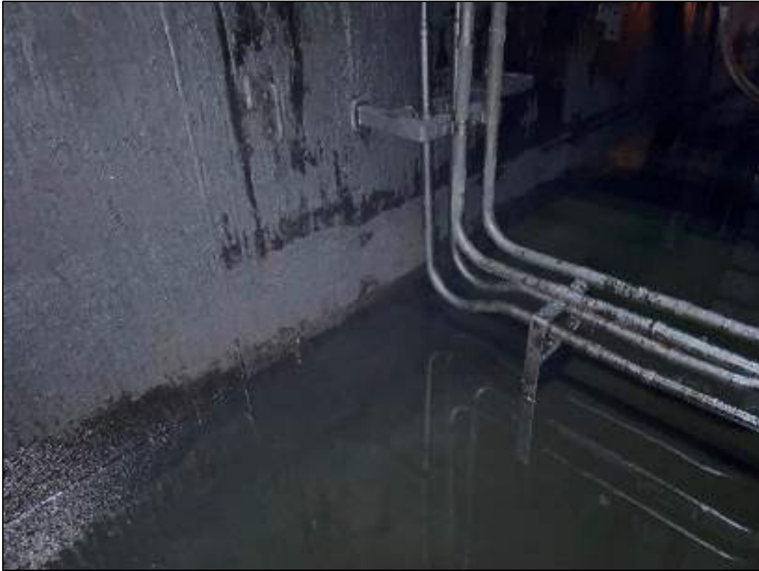
Figure 13: Firefighting water inside the slop tank
