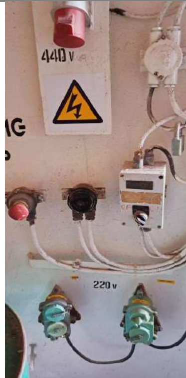
Figure 3: 220-V and 440-V sockets and the emergency stop for the crane located inside the pedestal of Crane No. 2.
