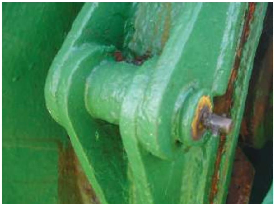
Ineffective grease point
