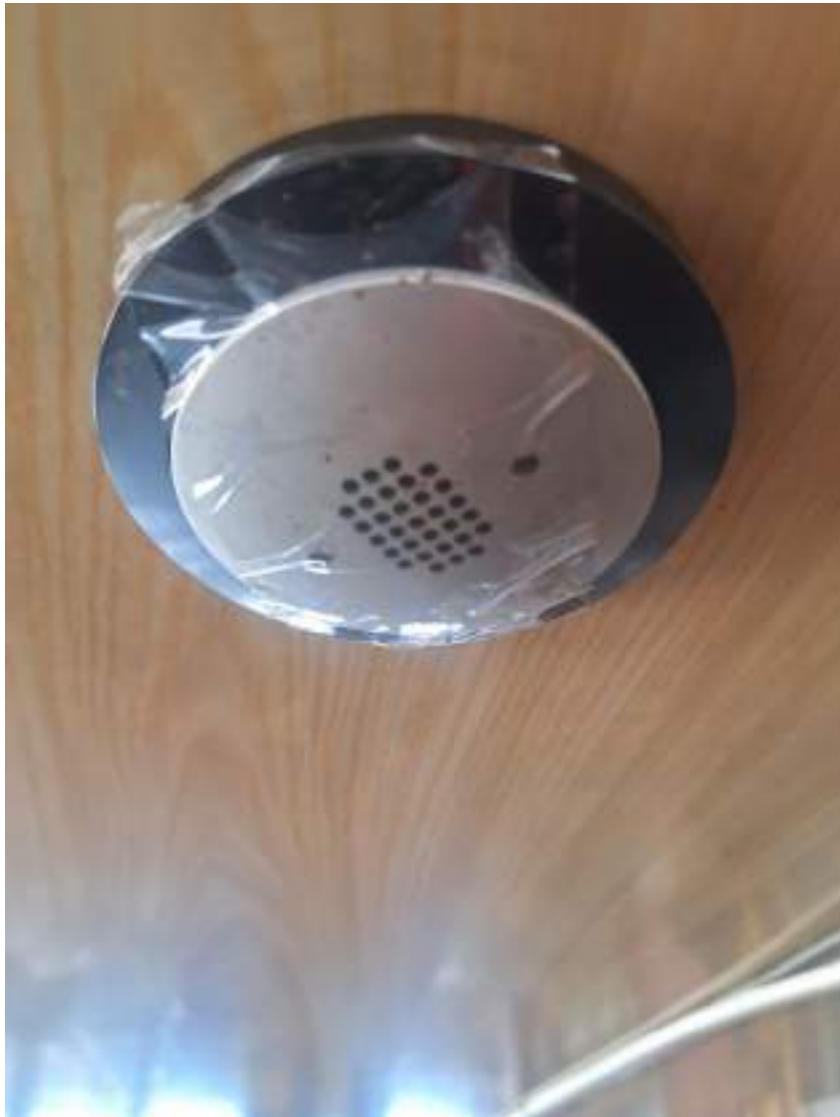
Bridge Speakers are Covered by Tape
