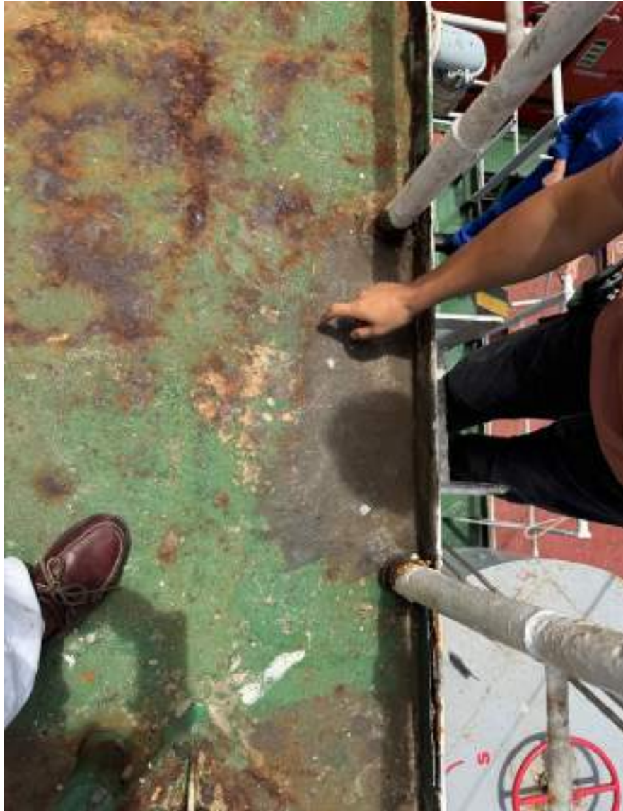
Heavy pitting on the monkey island deck - some areas have been patched up with fiberglass
