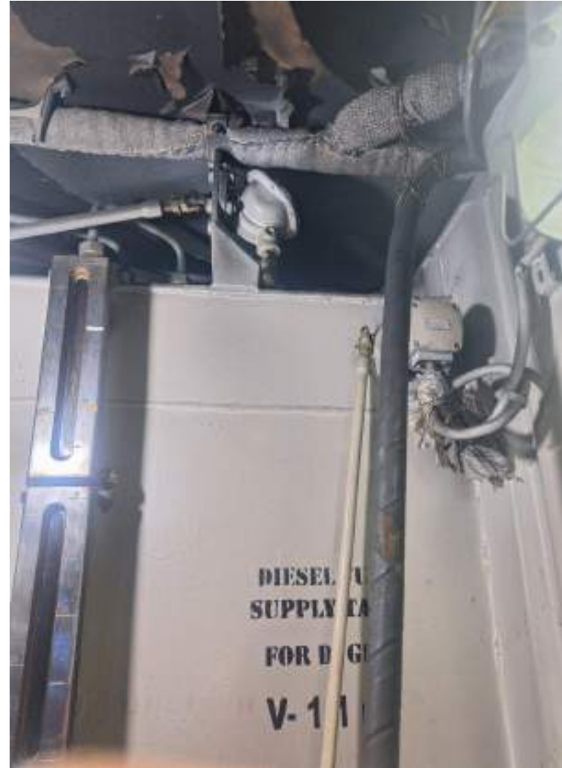
Quick Closing Valve of Diesel Generator Service Tank Disconnected
