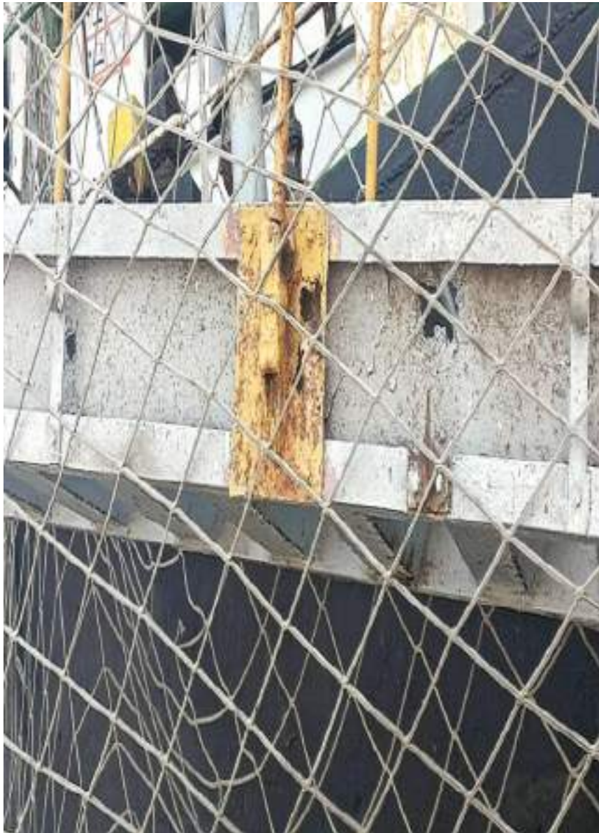
Accommodation ladder has some holes in the ladder construction
