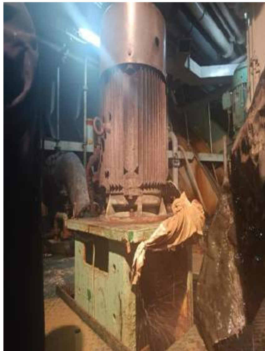
Fire / GS pump leaking extensively
