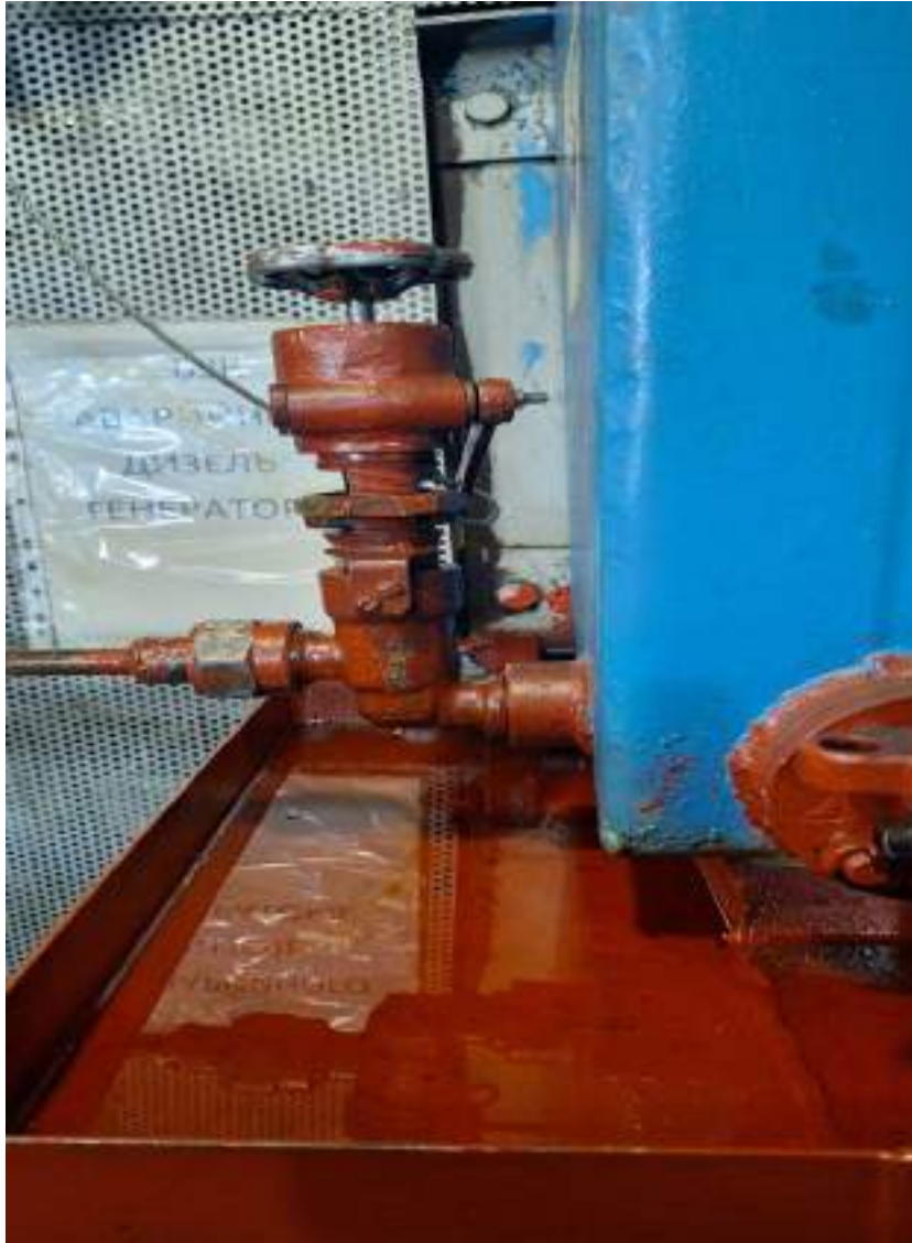
Quick Closing Valve of Emergency Diesel Generator Fuel Tank Leaking
