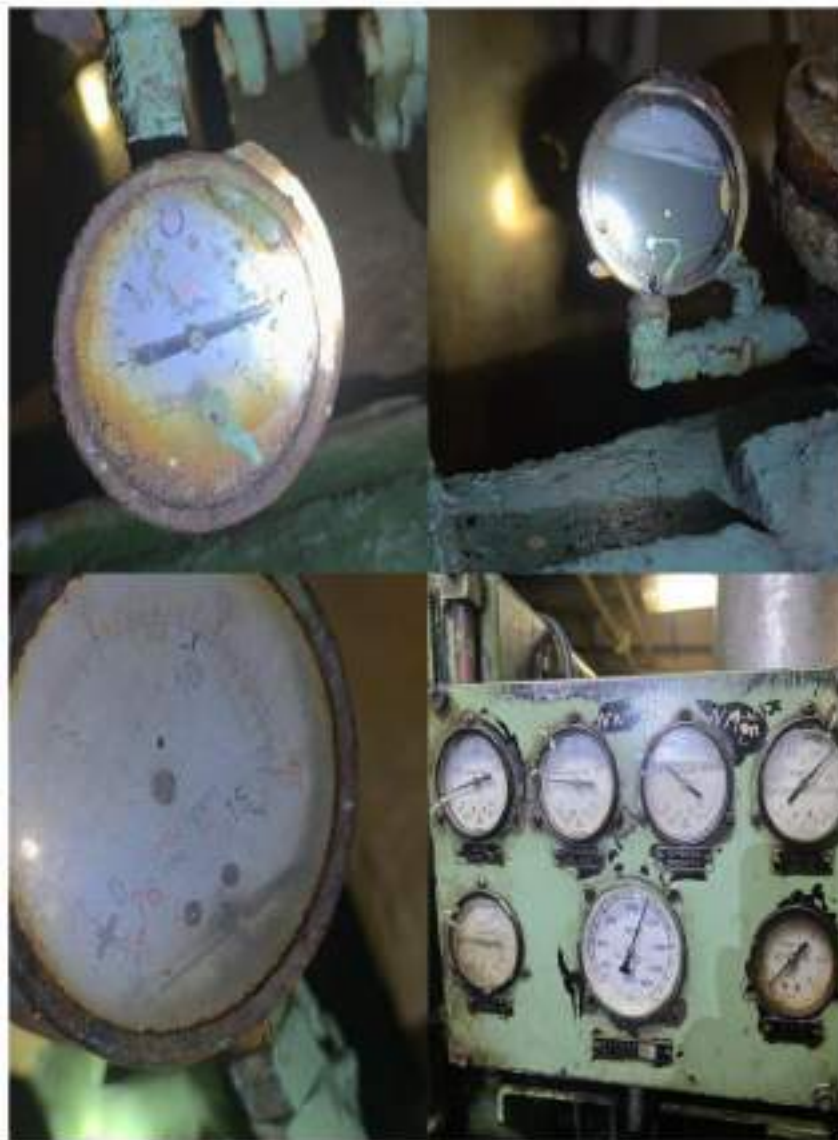
Gauges from cooling seawater pumps inoperative
