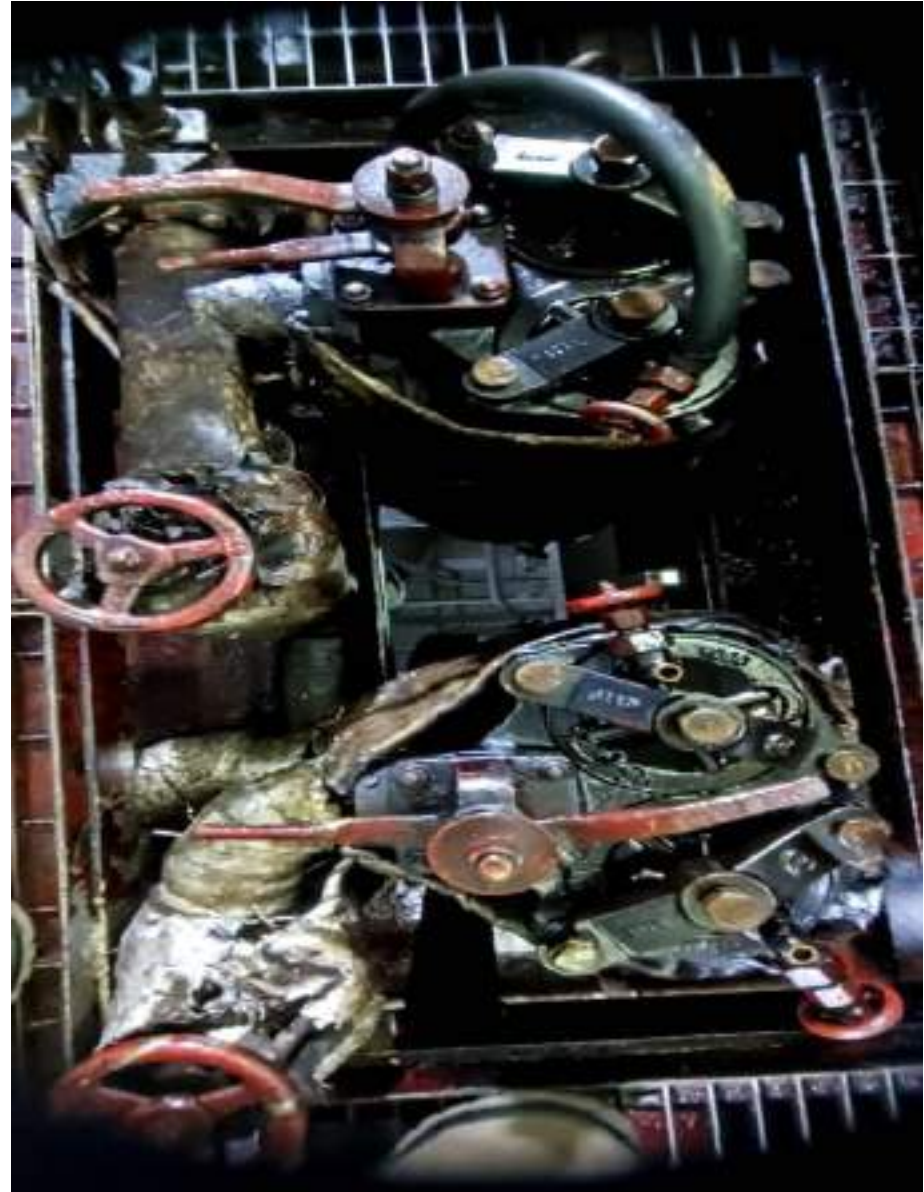
Oil accumulated in the engine room and steering gear room
