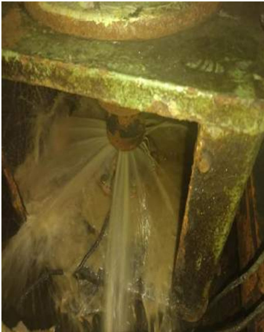
main cooling seawater pump leaking extensively
