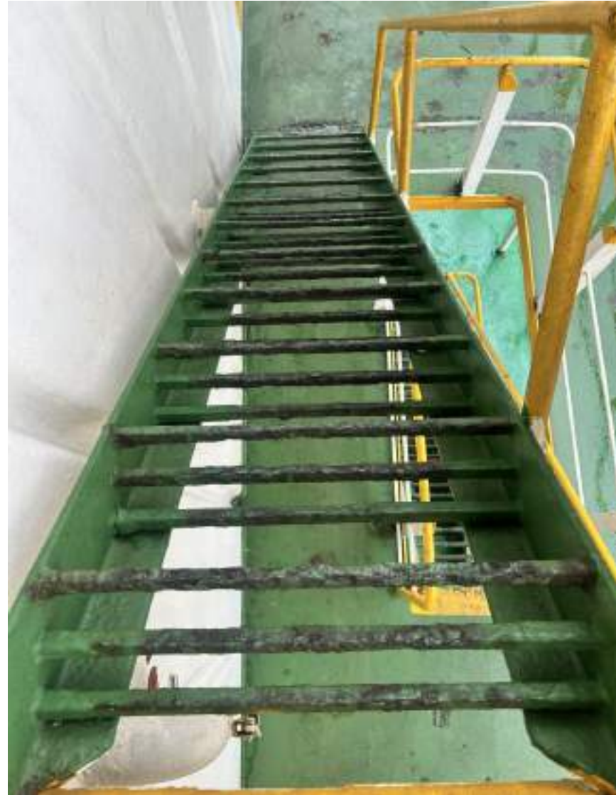
Life Boat's Deck's ladder's steps are rusty and unsafe
