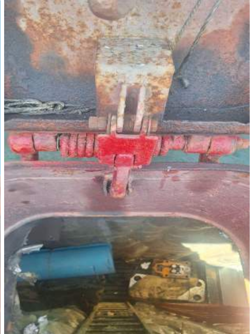
Safety Locker of Engine Room Emergency Exit Door in Poop Deck Removed
