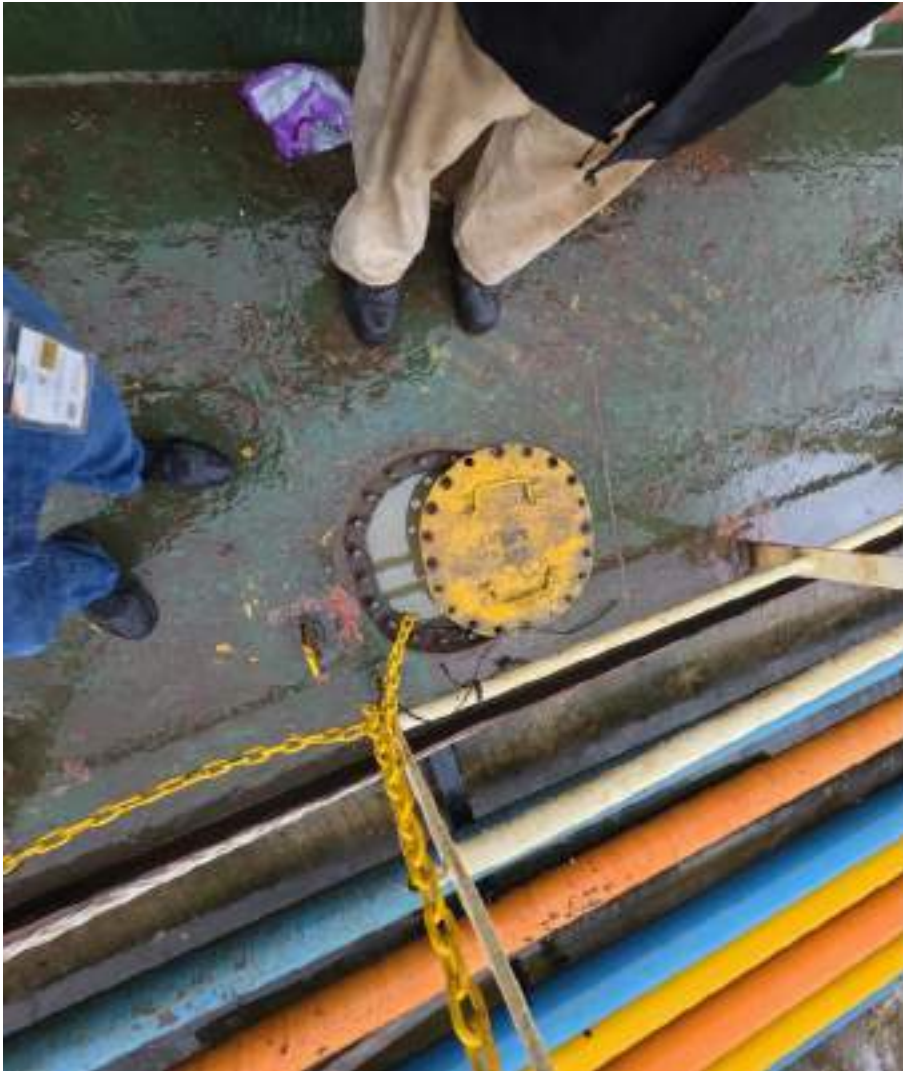
Water ballast tank sounding cannot measure by sounding pipes instead all ballast tank covers left open on deck to check sounding
