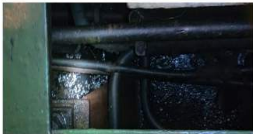
Oil and oily mixture found on tank top and bilge area
