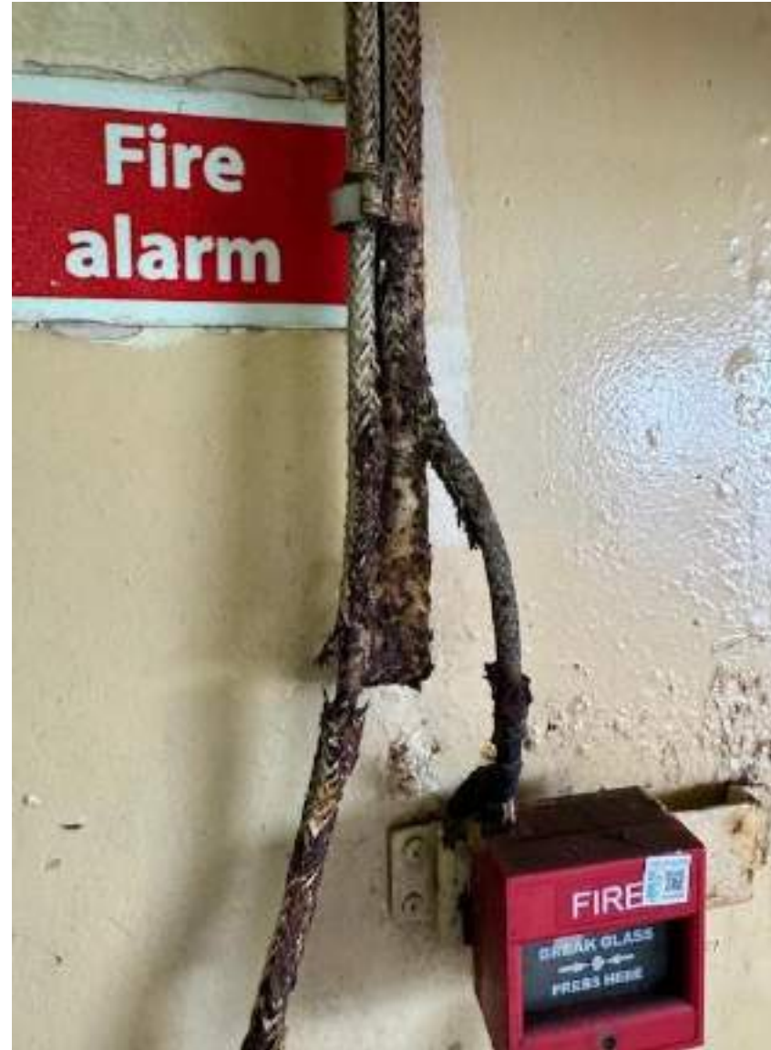
Electrical sockets around the accommodation in poor condition some of them are not even secured in the bulkhead
