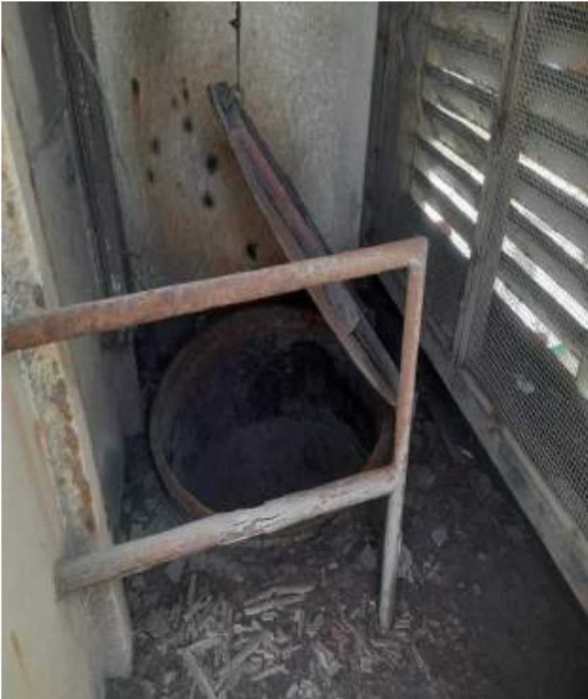
Both ER vent flaps are found corroded and with missing rubber packings
