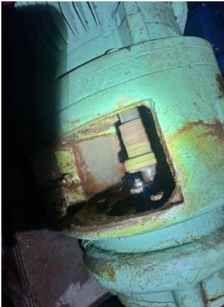
Service Cooling Pump for Generator was found leakage
