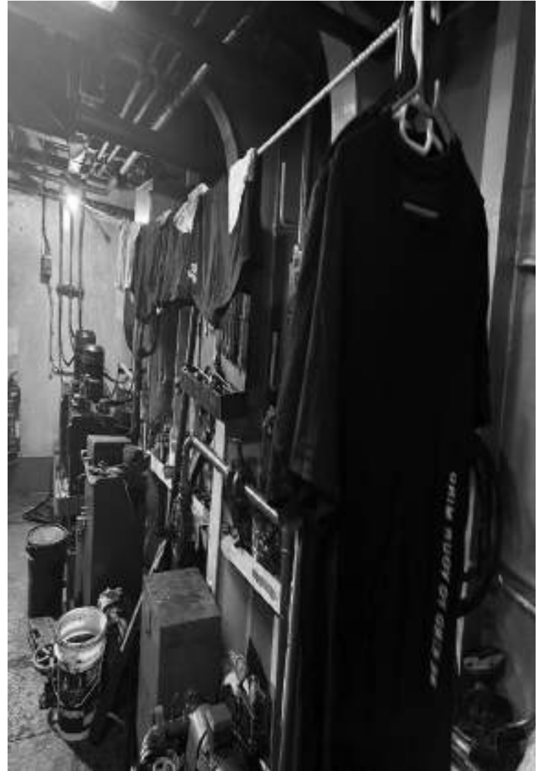
Engine room found with civil cloths hanging all over the place
