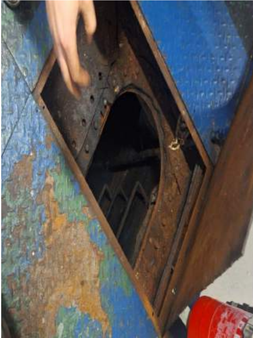
No Means Available for Sewage Tank Level Indication
