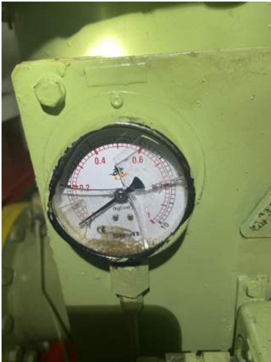
Lube oil Filter pressure gauge was found glass cover broken and defective condition
