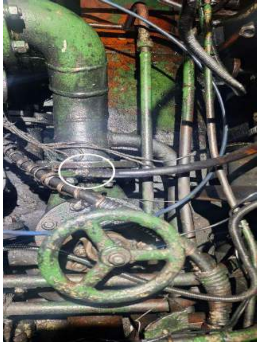
Fuel Leakage Line of STBD Side Main Engine not Connected to Tank and Fuel Leaking to Bilge
